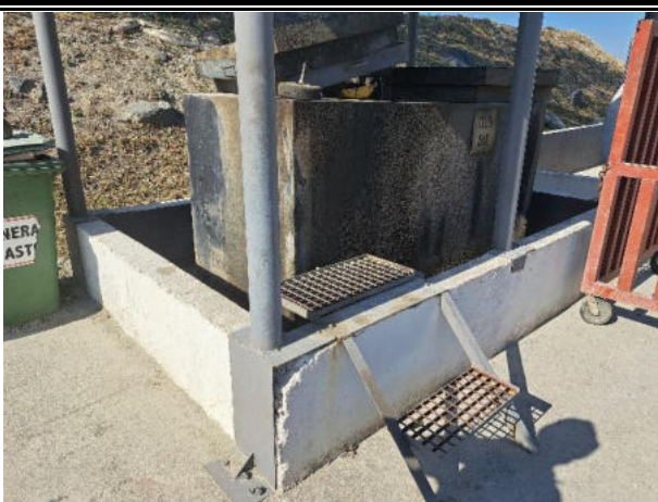
Used oil tank bund to be sealed
