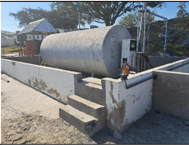
Diesel tank bund wall to be sealed
