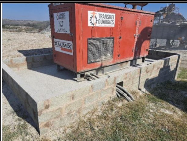
Generator bund to be sealed
