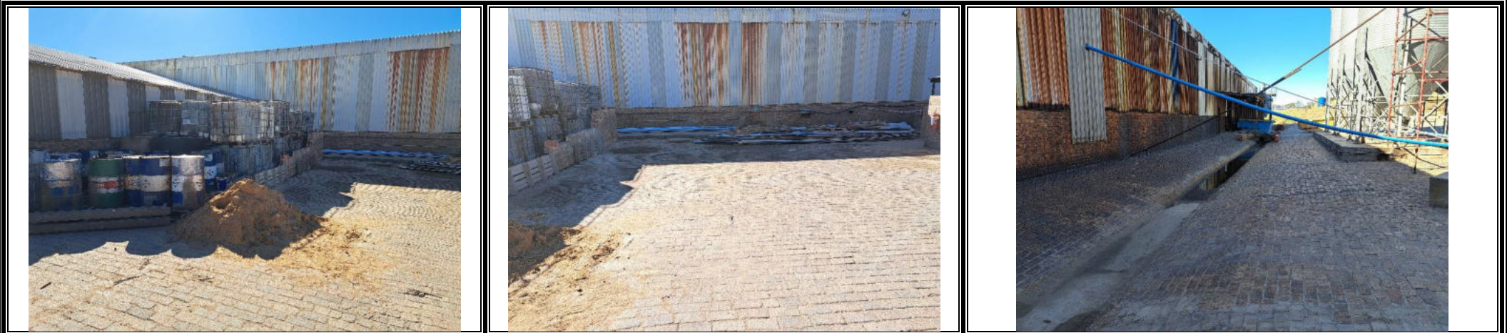
Bund of the used oil containers to be finalised to prevent dirty water runoff entering the nearby stormwater channel
