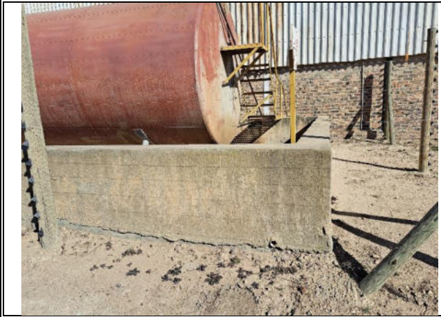
Bund to be sealed
