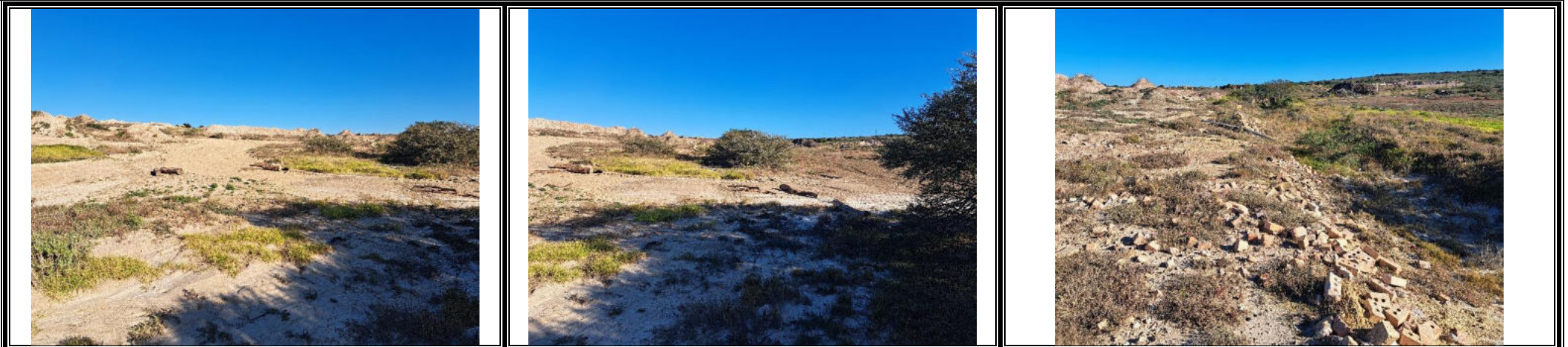
Drainage channel blocked by a road – to be opened and discarded bricks to be removed
