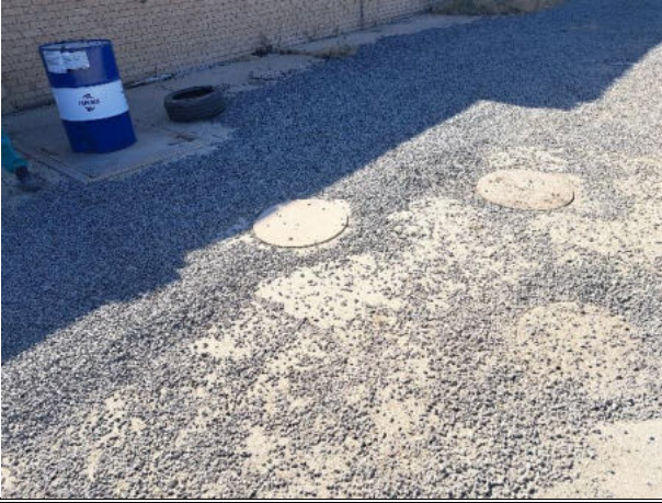
Oil sump of the wash bay
