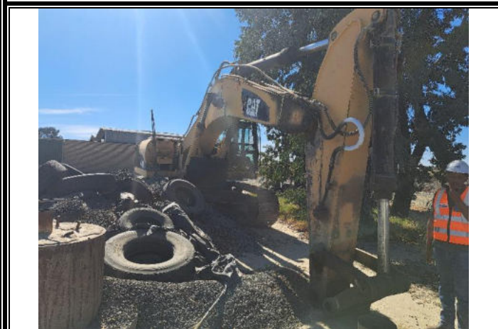
Machine to be repaired and/or removed from site. Spills to be cleaned
