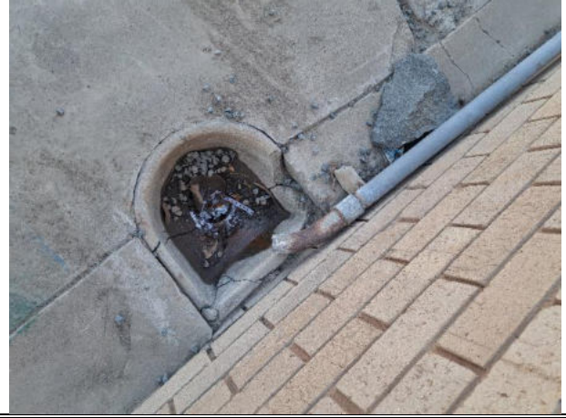
Drain to be cleaned
