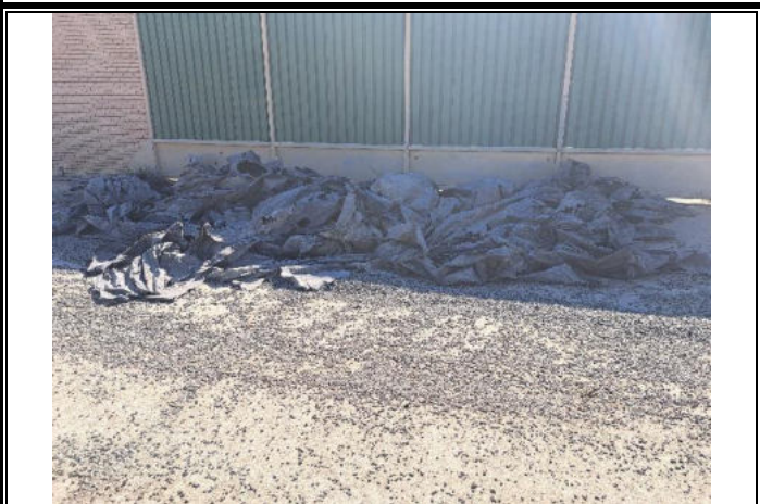
Old bags/plastic to be removed from site
