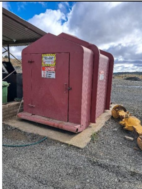
Oil store with build in bund
