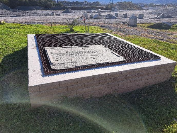
Last chamber of the oil sump
