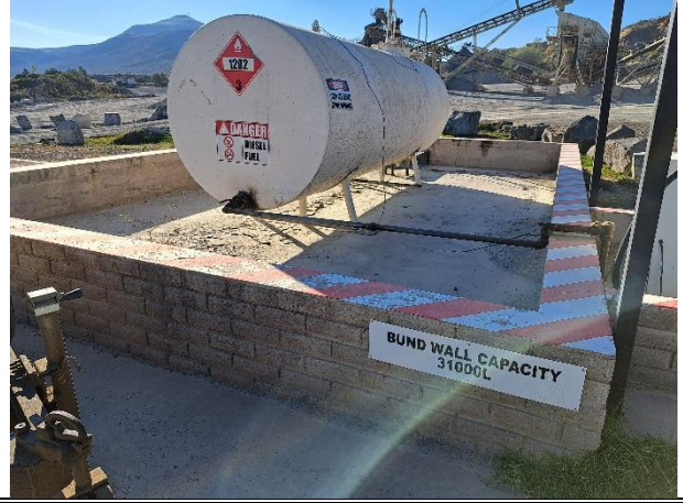
Bund of the diesel tank to be sealed
